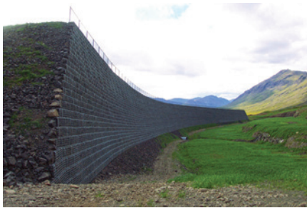
Avalanche barrier - Neskaupstaður (Iceland)
