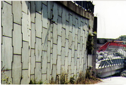
Izmit earthquake (Turkey)
